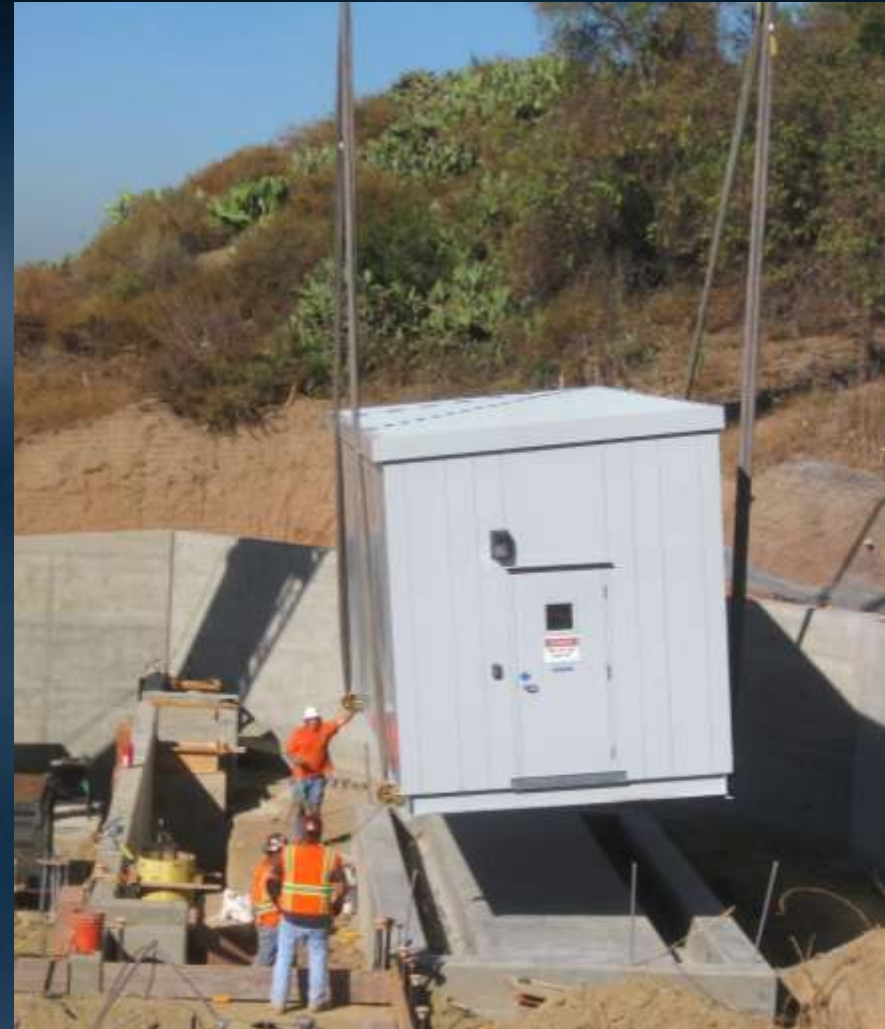
Motor Control Center placement
