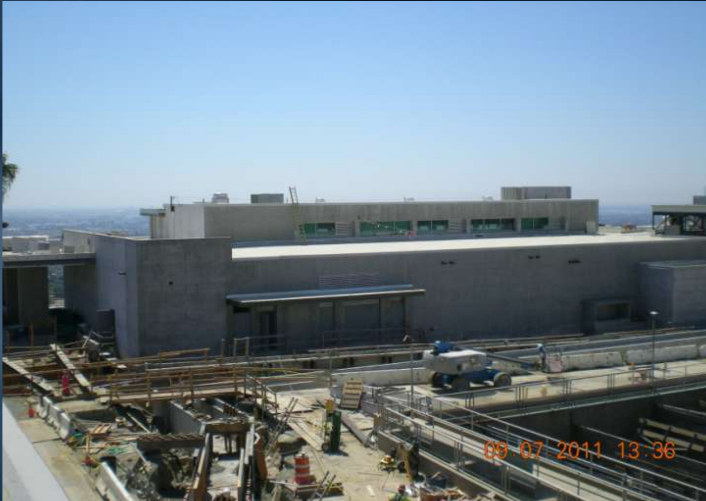
Ozone Generation Building
