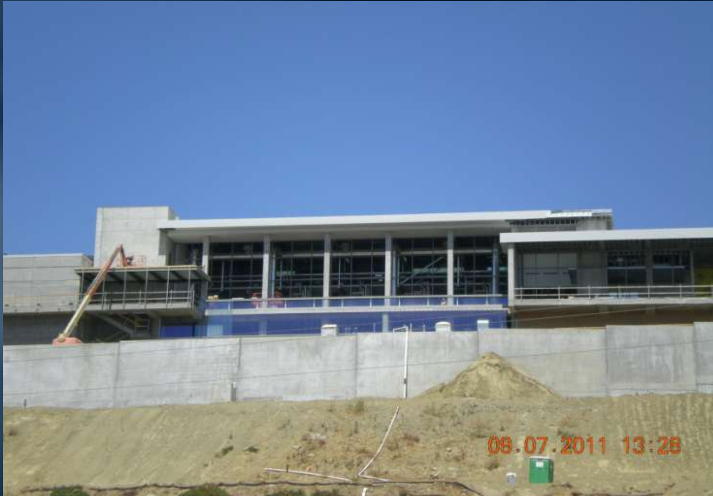
Ozone Generation Building
