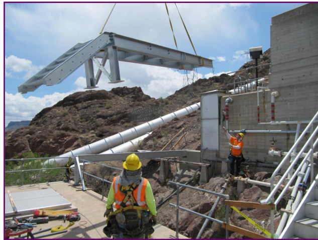
Colorado River Aqueduct Access Covers and Water Tank Improvements—Setting of the water tank platform at Intake Pumping Plant
