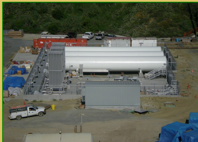
Diemer ORP – Liquid Oxygen Tank Farm
