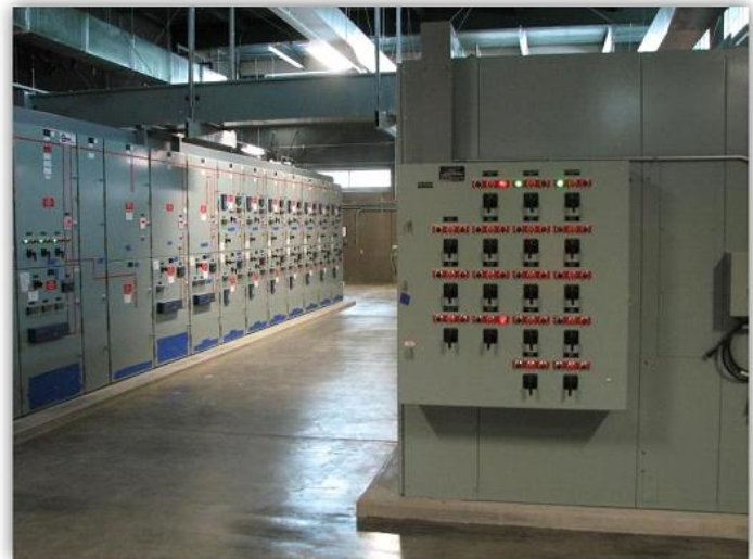
Diemer Treatment Plant New electrical switchgear
