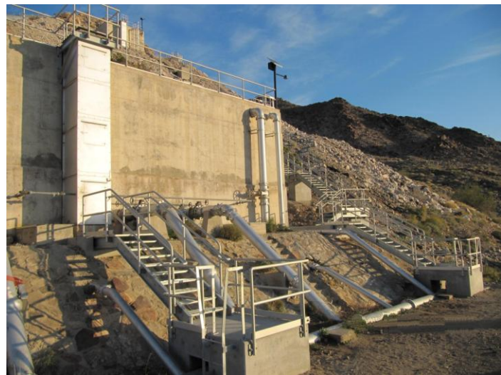
CRA Access Covers and Water Tank Improvements New landings and stairs at one of the circulation water tanks
