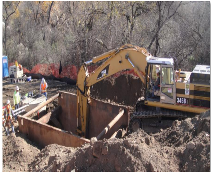
Box Springs Feeder Refurbishment - Phase 3 Shored excavation at one of the replacement sections
