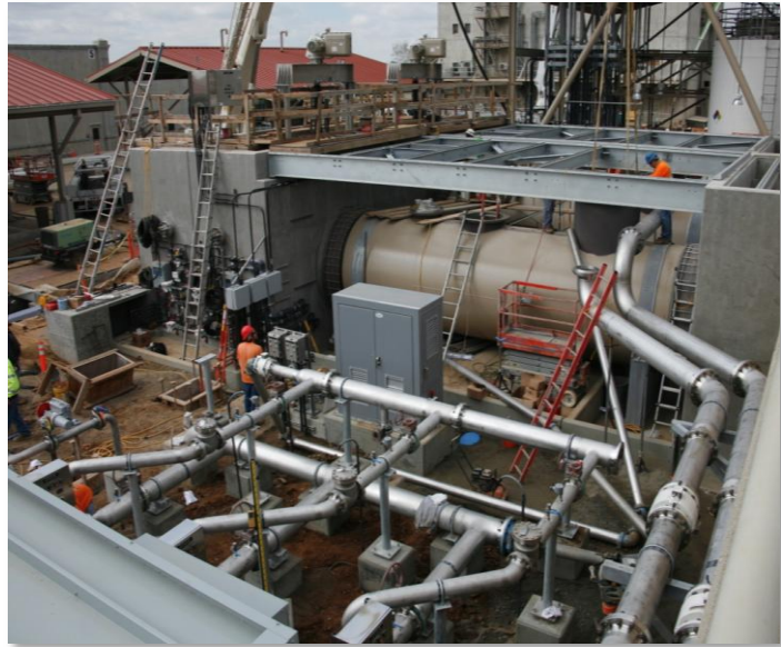
Weymouth Treatment Plant Testing and start-up of the new rapid mix system
