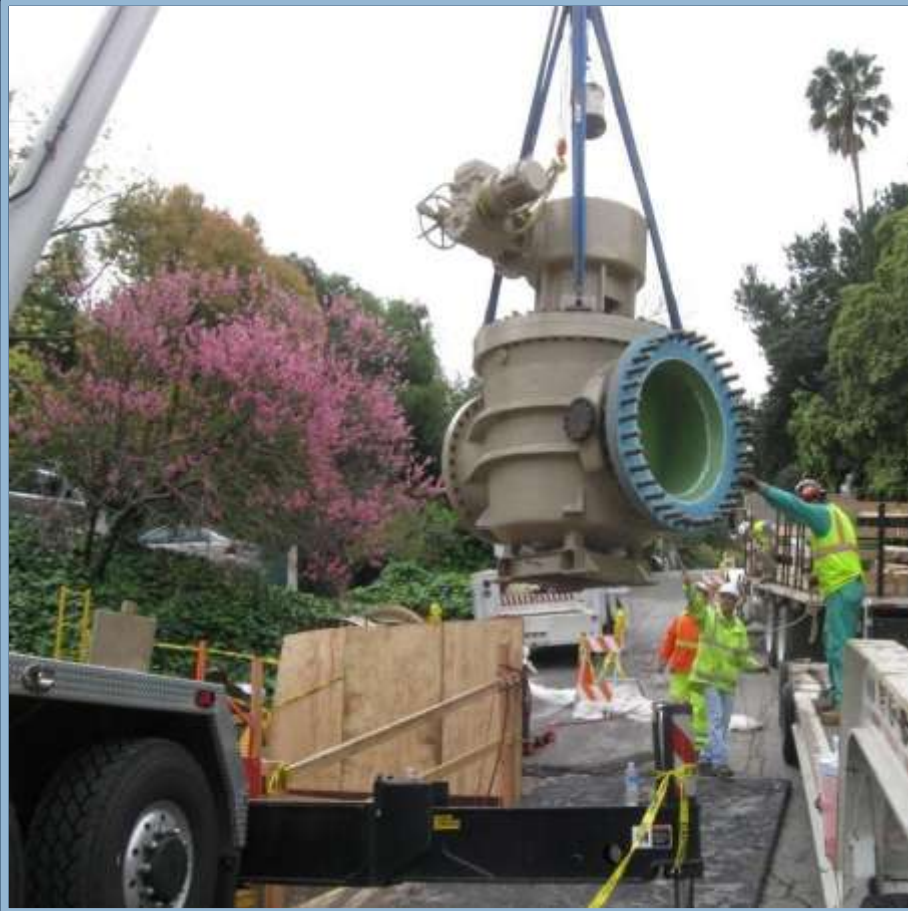
Unloading valve at site
