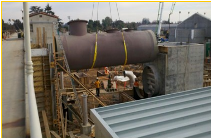
Weymouth Inlet Conduit Relocation Construction of 96-inch basin inlet pipe (Story on page 2)
