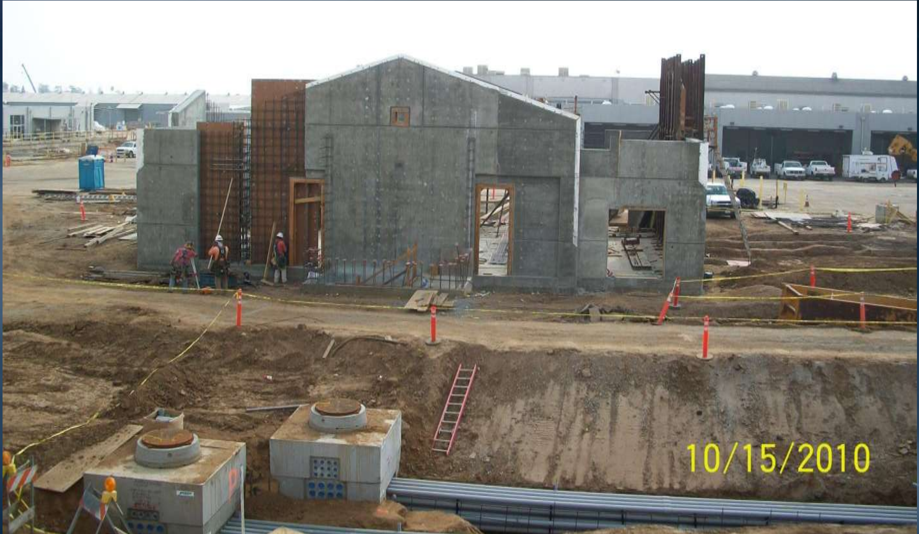
Main Plant Switchgear Building
