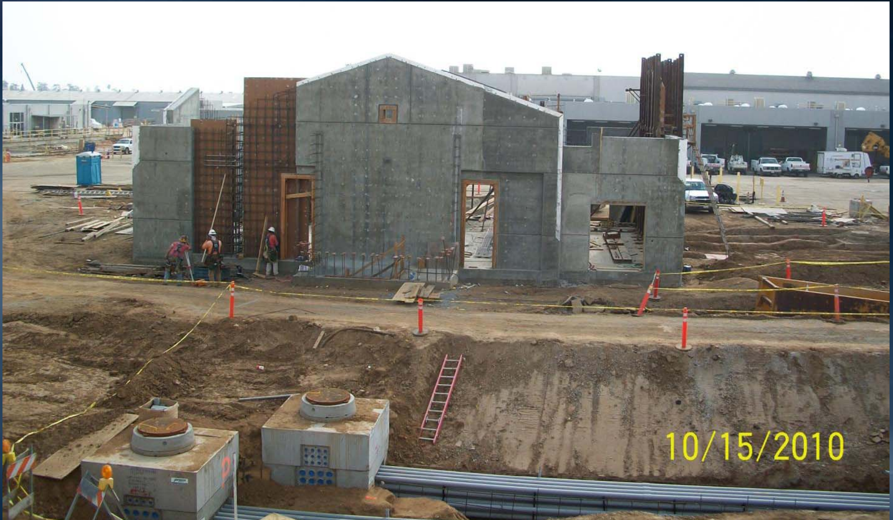
Main Plant Switchgear Building
