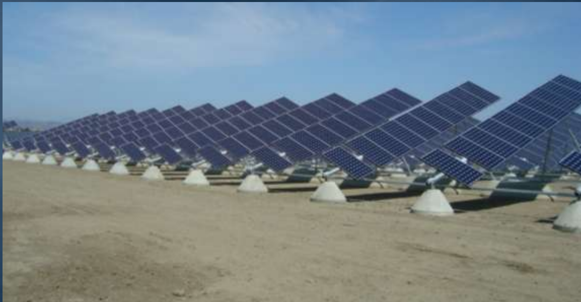
Skinner Solar Facilities
