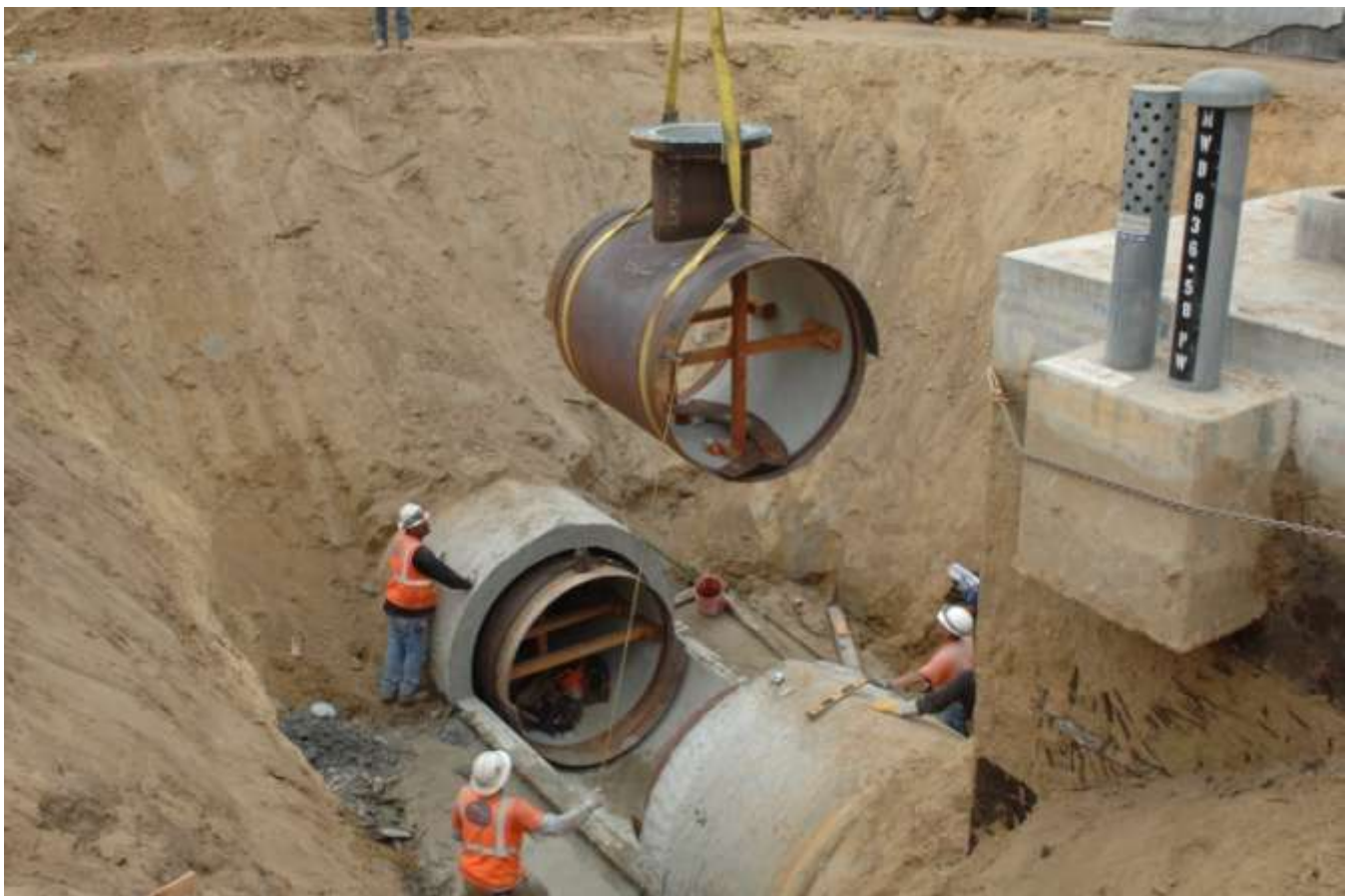
Figure 1: Installing new steel liner inside the existing PCCP line on the AMP
