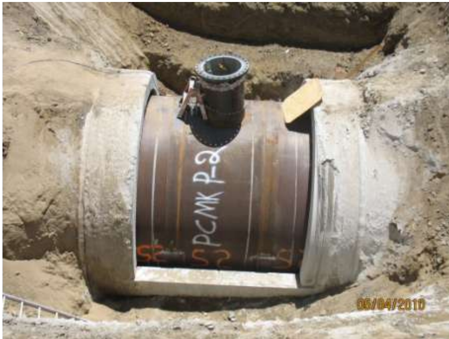
Figure 3: New steel liner inside the existing PCCP line on the Lake Skinner Outlet Conduit
