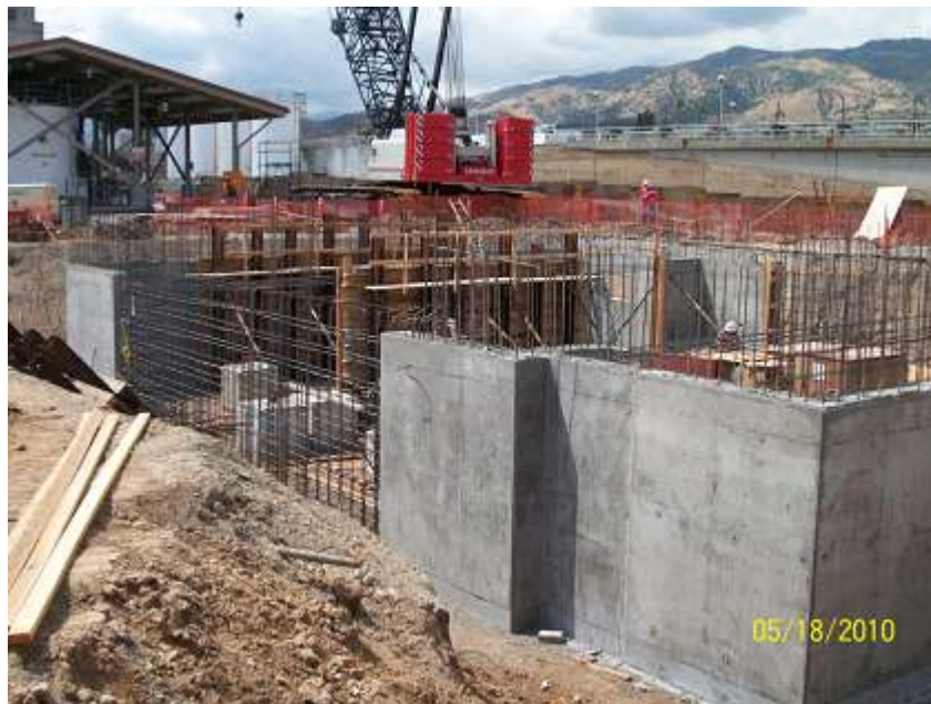
Figure 5: Construction of the main plant switchgear building for the Weymouth Electrical Upgrades
