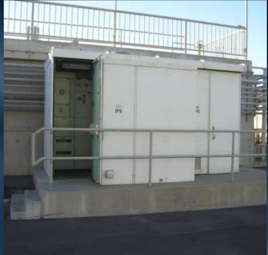
Typical MCC Building
