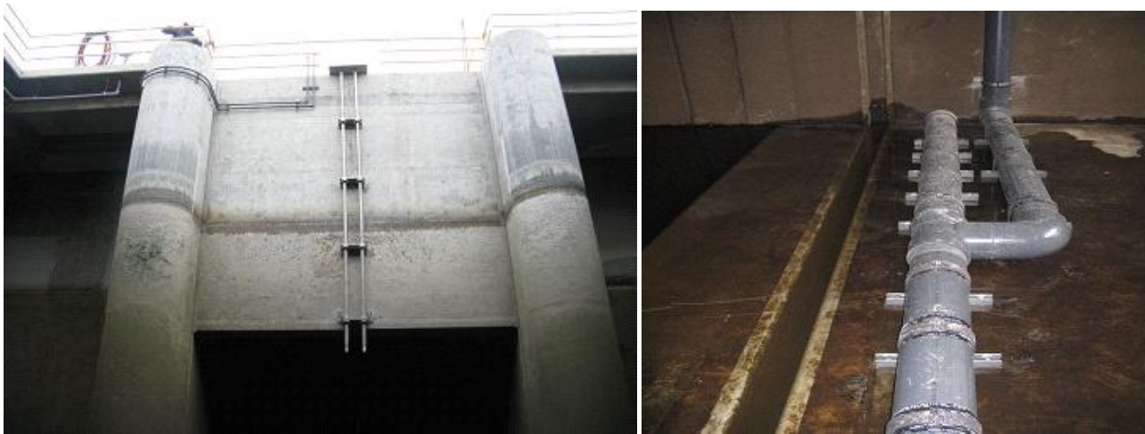
Figure 4: Left: New ammonia injector. Right: New chlorine injector
