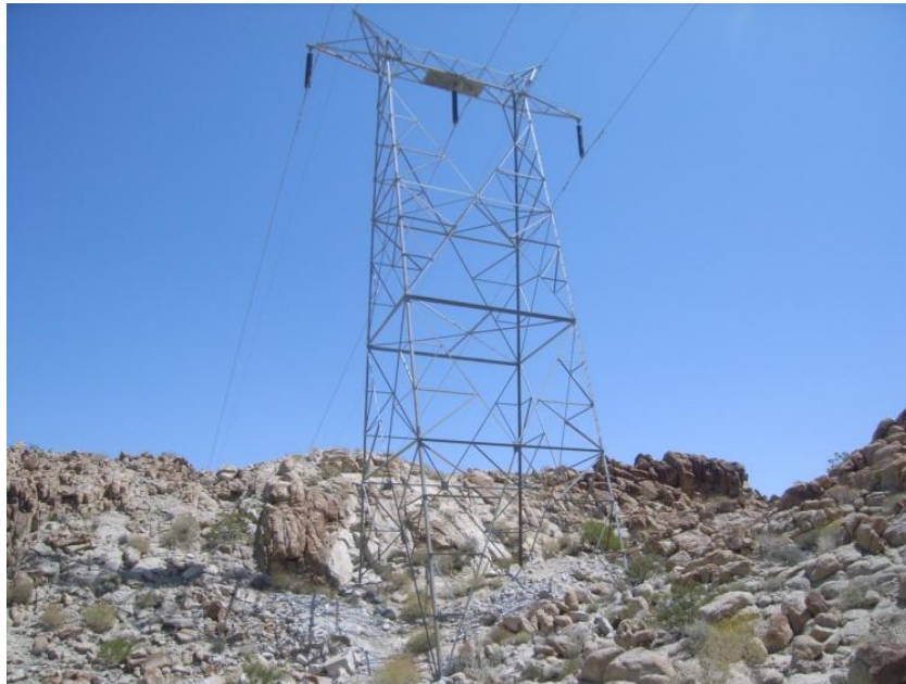
Figure 10: Metropolitan transmission tower
