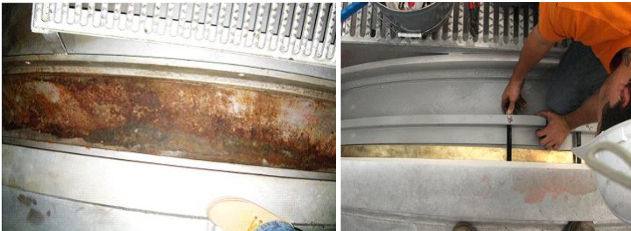
Figure 5: Left: Leaky expansion joint before repairs. Right: The same joint following completion of repairs.
