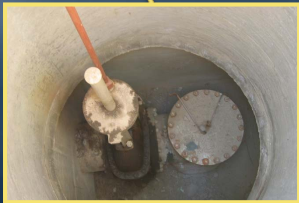
Leaky 1950s gate valve
