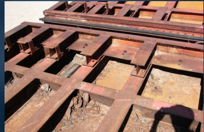
Corroded isolation gates
