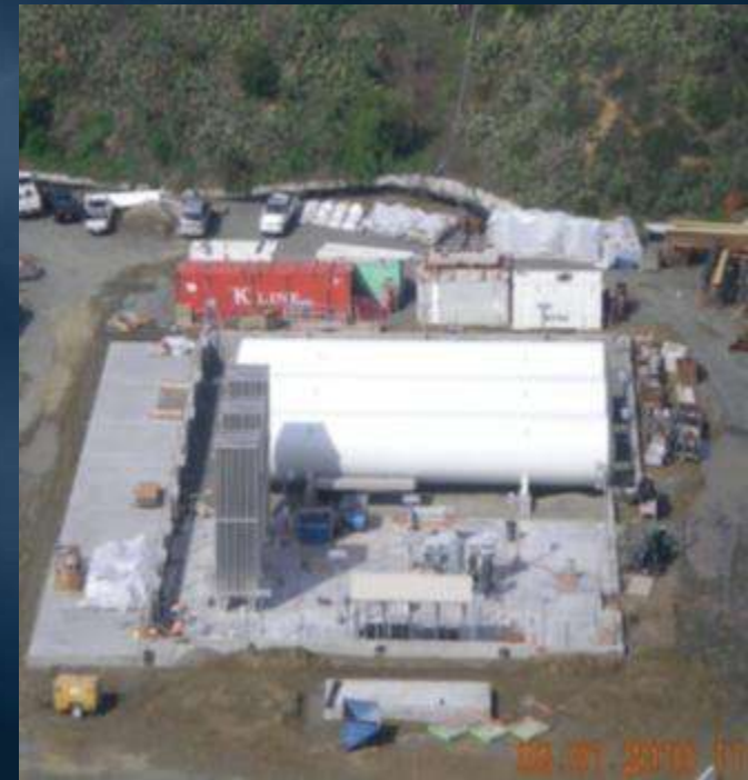
LOX Tank Farm
