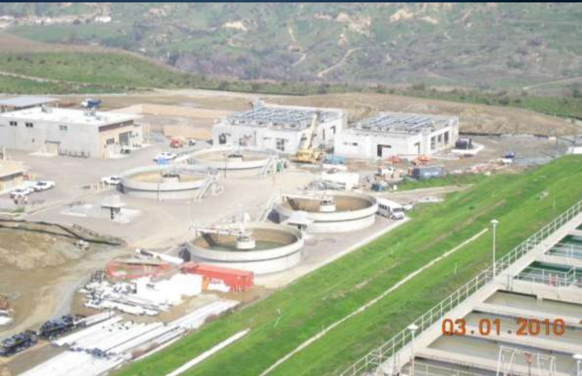
Switchgear Building and SCE switchyard Upper Pad
