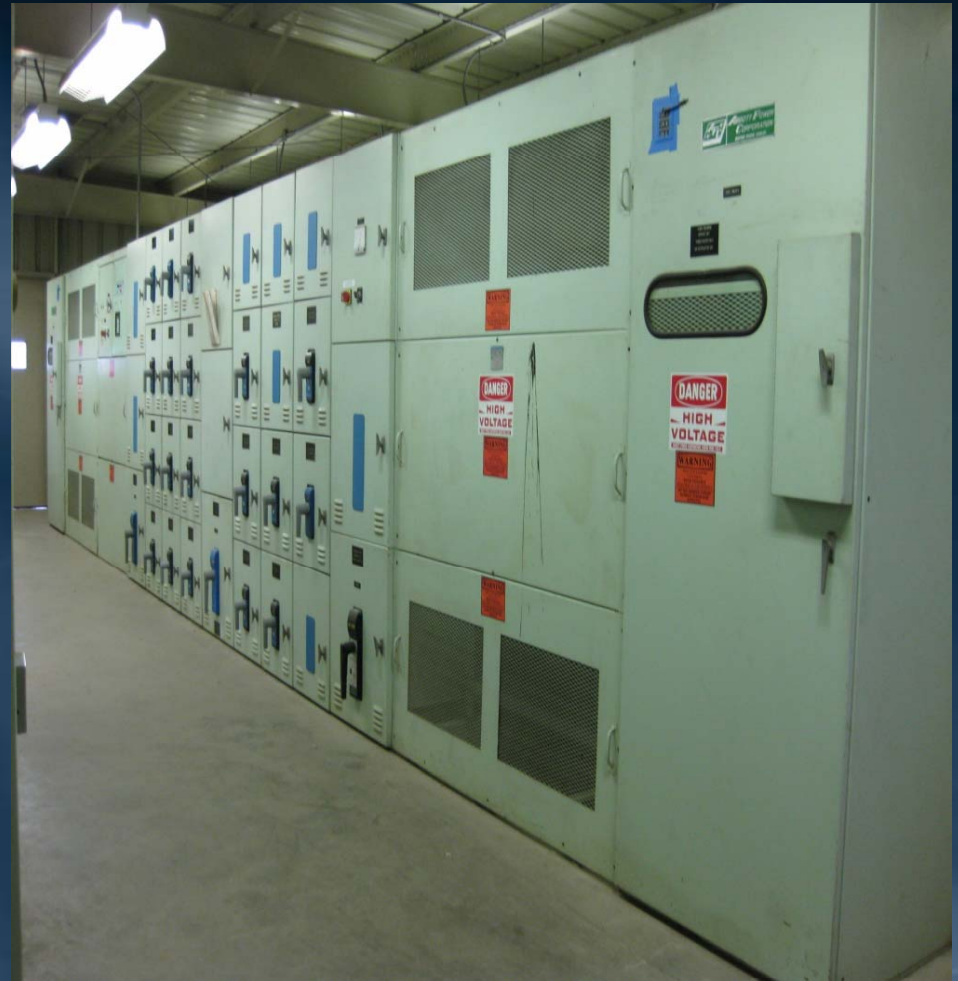
Unit Power Center
