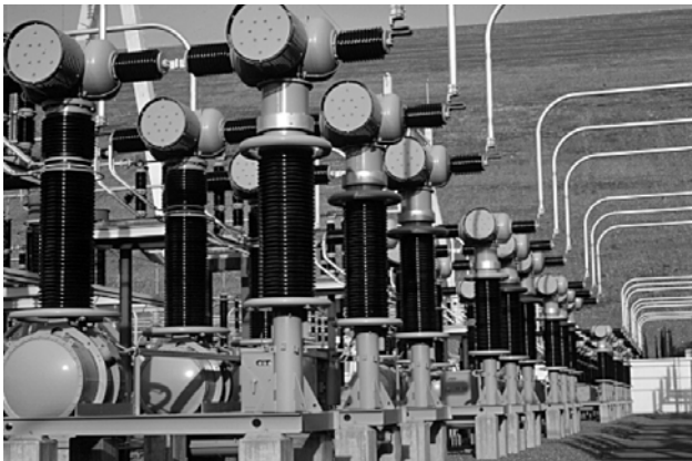
Figure 2. Close-up of Hyatt Power Plant switchyard (DWR Photo).
