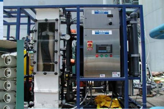
Memcor Microfiltration Unit
