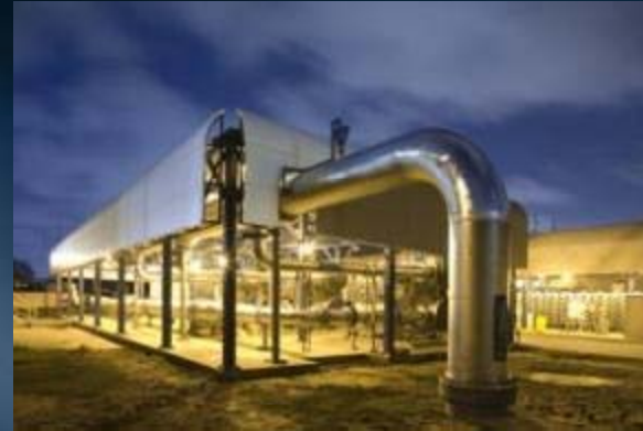
Edward C. Little Water Recycling Facility
