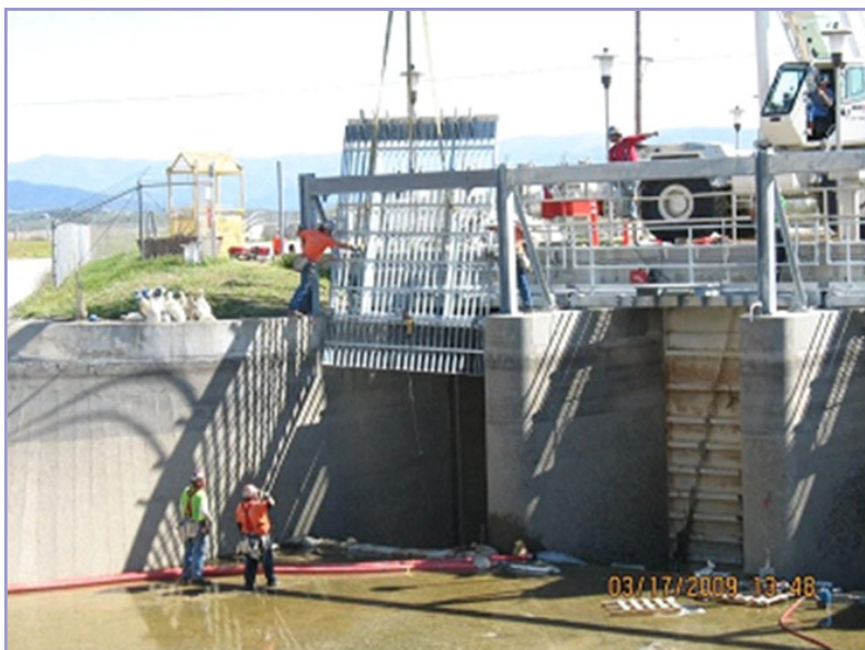
Lake Skinner East Bypass Screening Structure Rehabilitation—Installation of new trash racks at bypass entrance.
