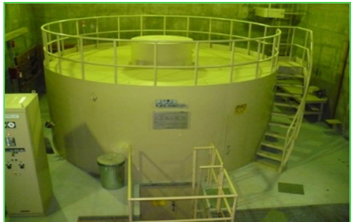
System Operations—Lake Mathews Hydro Electric Plant
