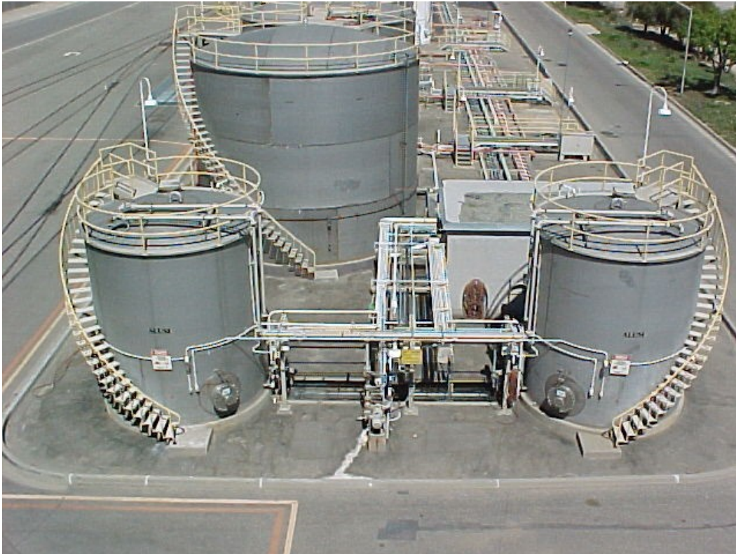
Figure 9: Jensen Caustic Tank Farm
