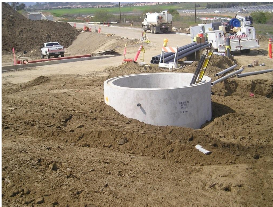
Figure 7: New chlorine injection manhole
