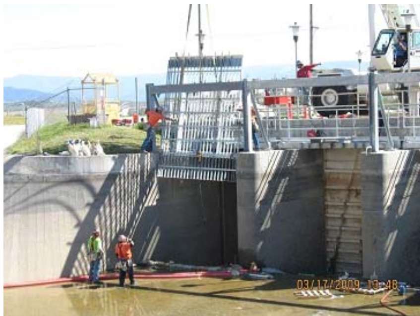
Figure 5: Installation of new trash racks at Lake Skinner East Bypass Screening Structure.
