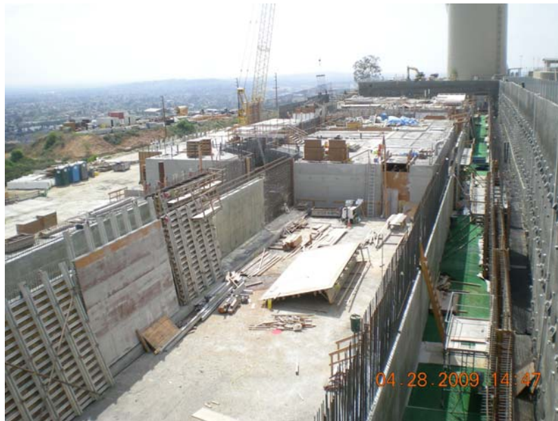
Figure 10: Diemer ORP Ozone Generation Building and Contactors
