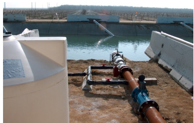
Figure 6. Semitropic arsenic treatment demonstration program (MWD photo.)
