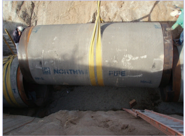
Perris Pipeline—Installation of the final pipe segment for Perris Valley Pipeline North Reach
