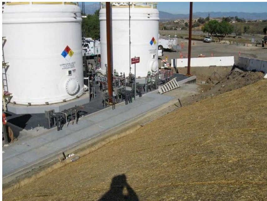
Figure 4: Lake Mathews Interim Chlorination Facility
