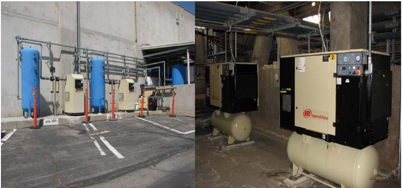
Figure 6: Weymouth air compressors (former equipment on left, and indoor replacement equipment on right)
