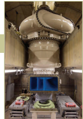
Pump at Edmonston Plant
