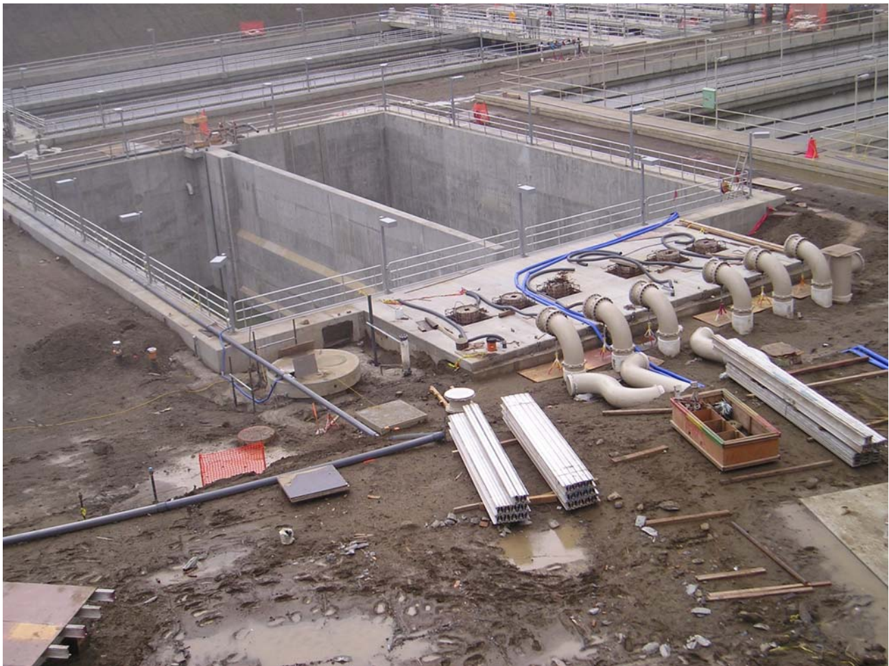
Figure 6: Skinner Reclamation Washwater Pumping station
