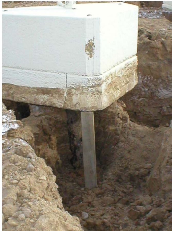
Figure 8: Soil excavation of the foundation piles for the purpose of evaluating their condition
