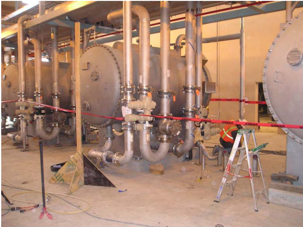
Figure 12: Installation of ozone generators at the Skinner plant
