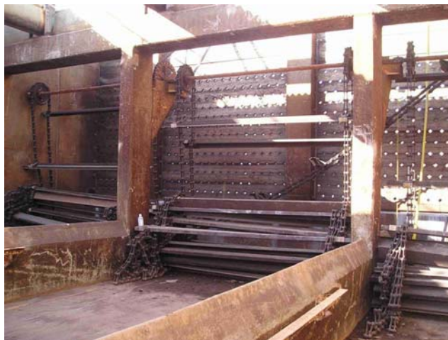
Figure 11: Washwater Reclamation Plant No. 2 existing solids collectors to be replaced
