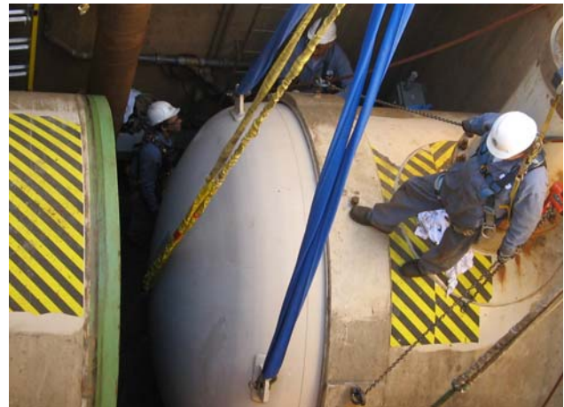
Figure 6. Installation of bulkhead to isolate the northern portion of the SAVP. (MWD Photo.)
