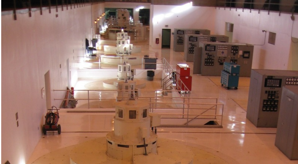
Figure 13. Pearblossom Pumping Plant. (MWD photo.)
