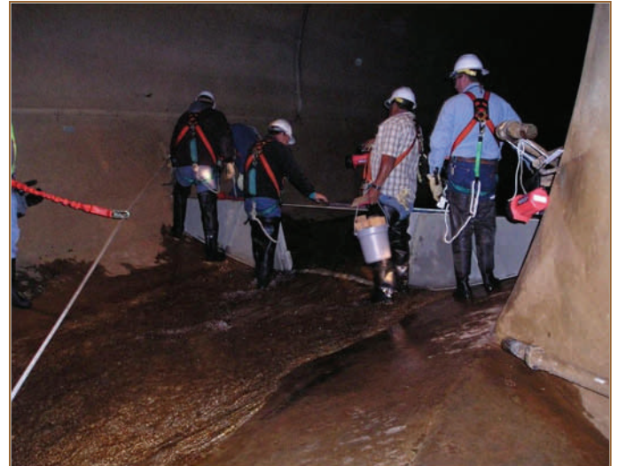
CRA Shutdown San Jacinto Tunnel Weir Measurement
