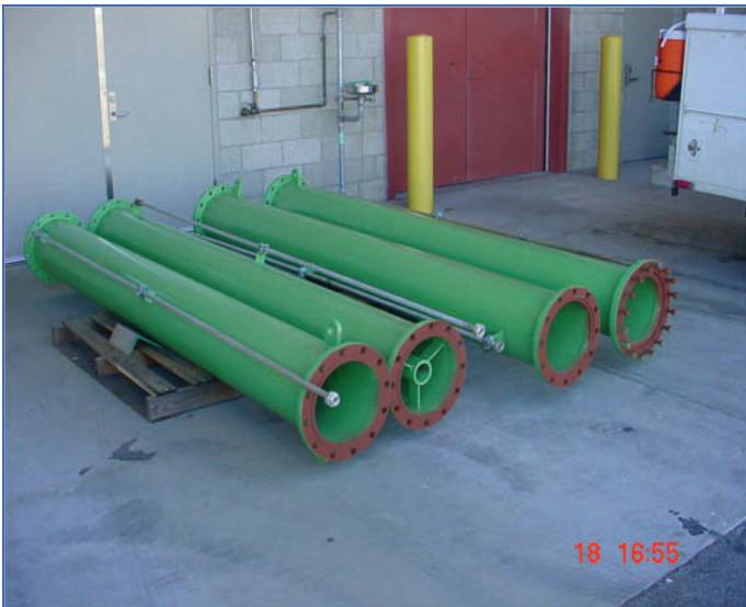
Prepped and coated pump columns for Jensen Washwater Reclamation Plant
