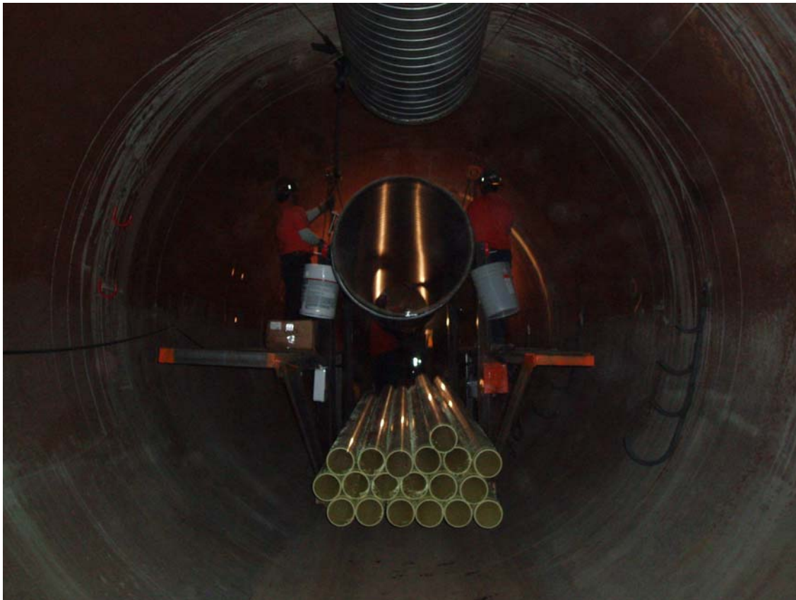
Figure 4: Installation of the ventilation lines in the City Creek portion of Arrowhead East Tunnel
