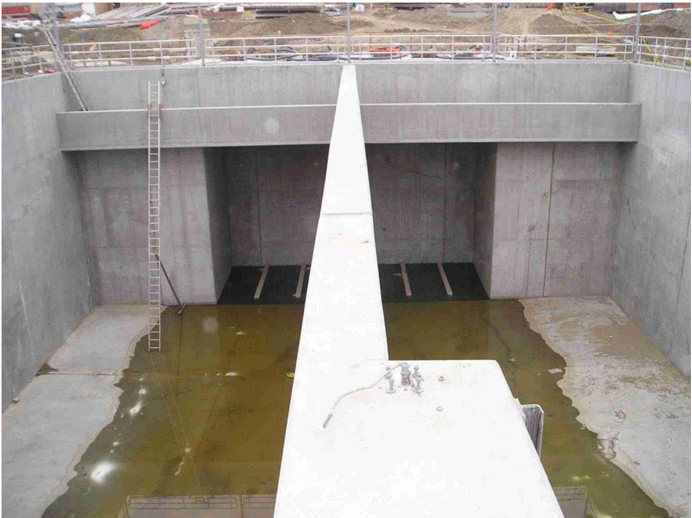
Figure 6: Skinner Reclaimed Washwater Pump Station
