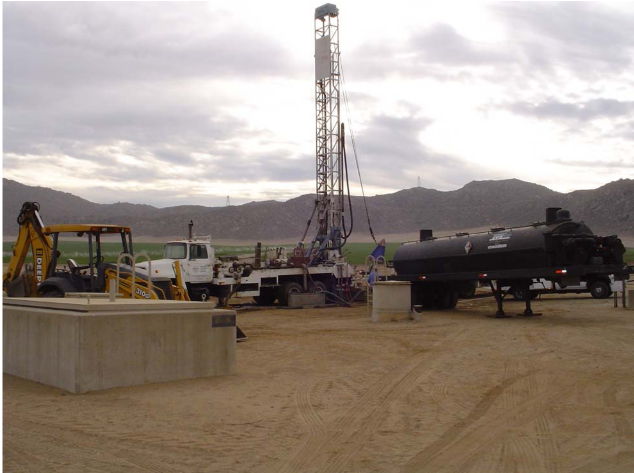
Figure 7: Installation of casing to connect anodes for cathodic protection of Lakeview pipeline
