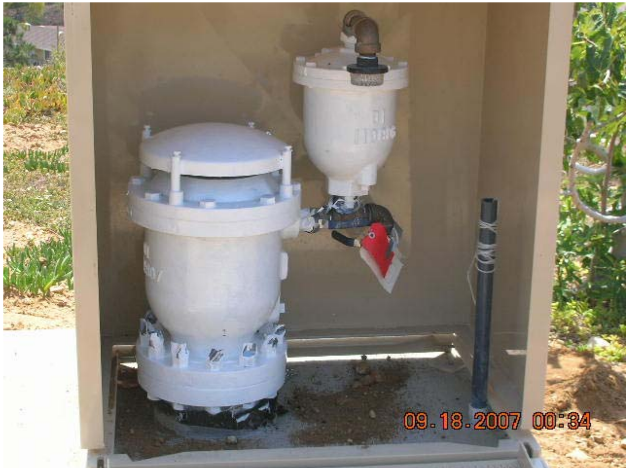
Figure 10: Air release and vacuum valve and enclosure
