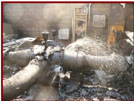
Fire damage at OC - 71 service connection
