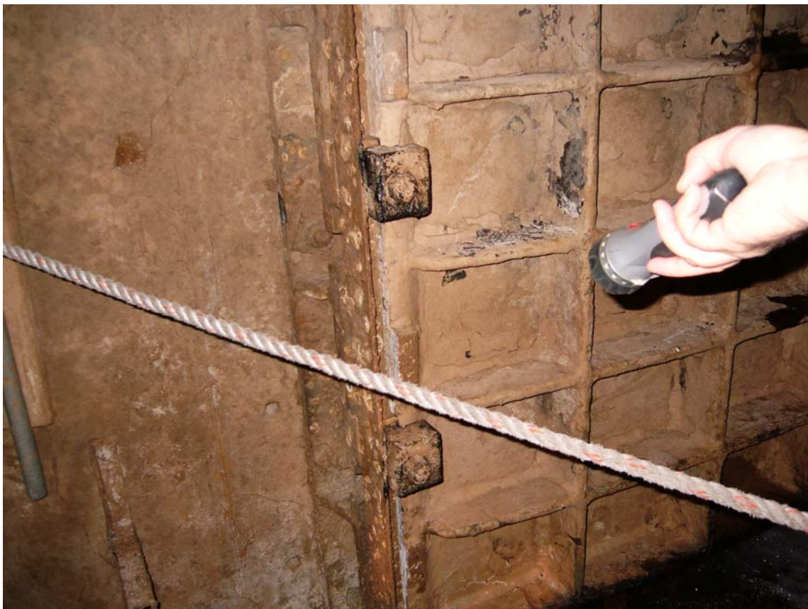
Figure 7: Corroded slide gates at San Jacinto Diversion Structure to be refurbished
