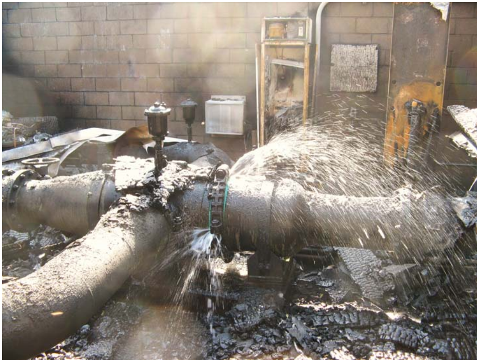
Figure 1: Fire damage at OC - 71 service connection
