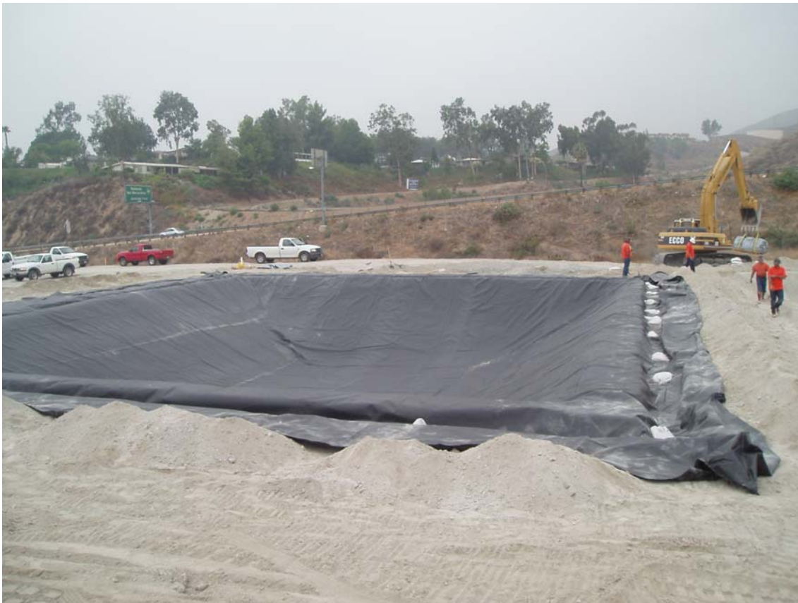
Figure 4: Arrowhead Tunnels installation of pond liner for the temporary tunnel discharge water treatment plant at City Creek Portal
