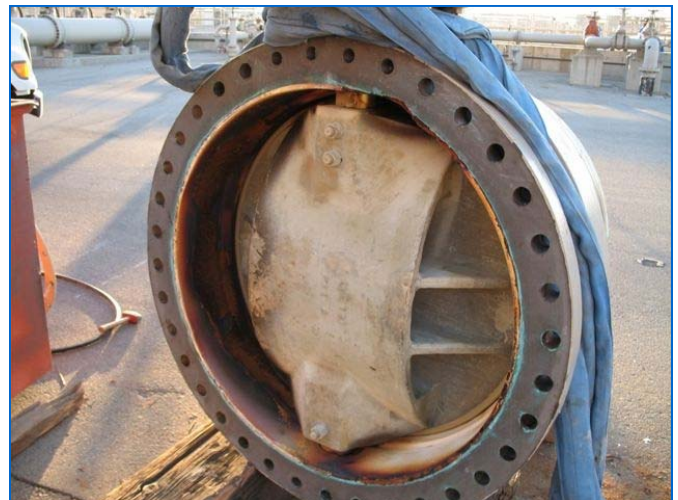
Backwash header valve
