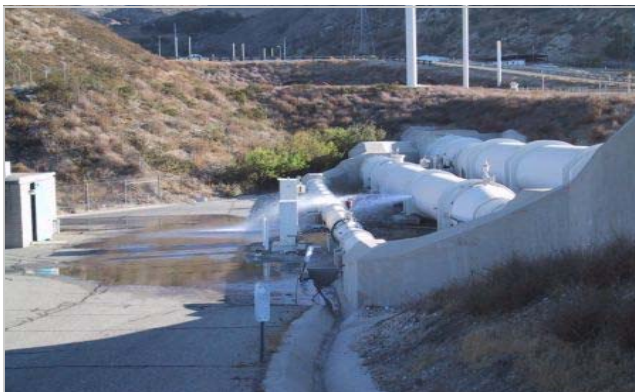
Rialto Pipeline Leak
