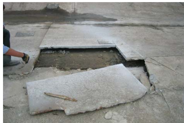
Concrete liner to be repaired in Orange County
