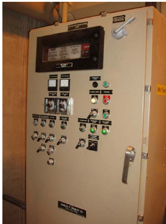
Figure 9: Dry polymer system control panel
