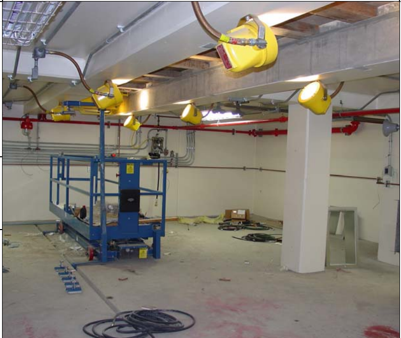
Installation of lights and vehicle lift equipment in lower level of new Vehicle Maintenance Center
