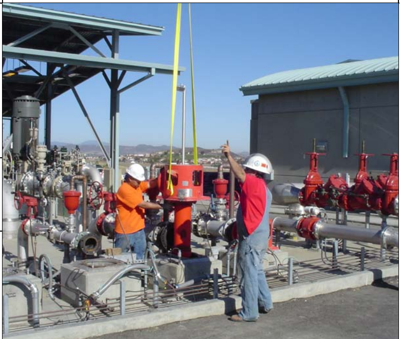
Removal of fire pump to exchange impellers at potable water pump station
