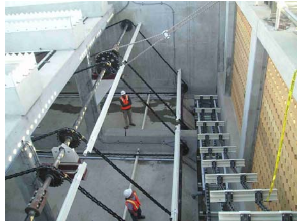
Solids Collection Installation
