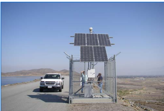
Installed new solar-powered surveillance cameras at Diamond Valley Lake where power connections are absent.
