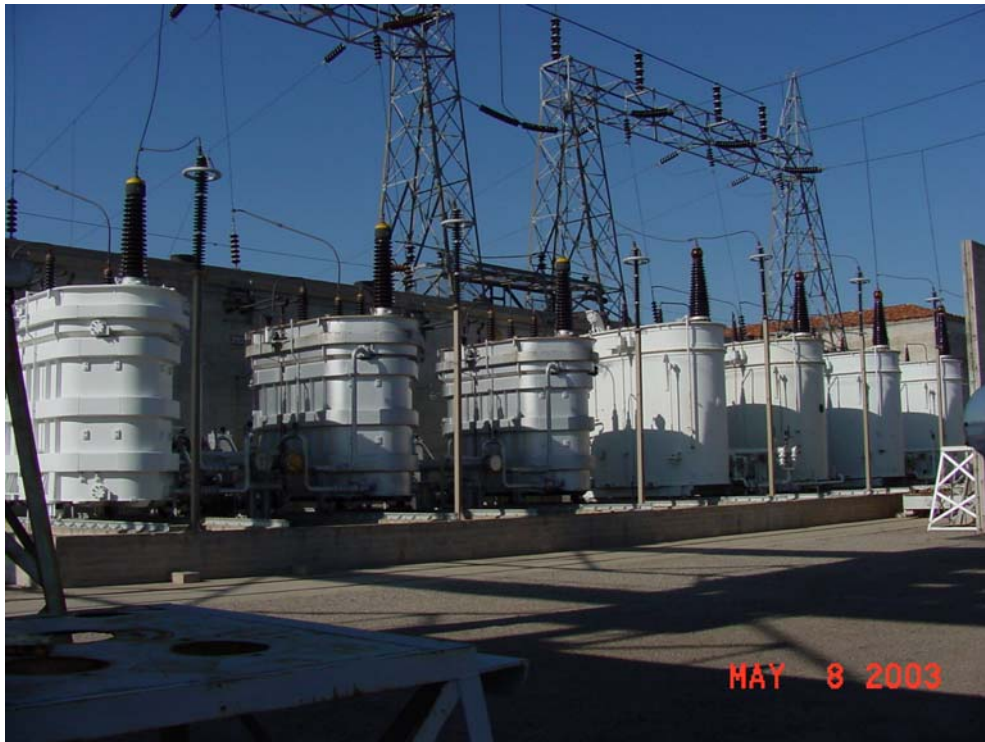
Figure 9: Transformers at Gene Pumping Camp
