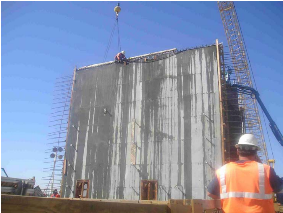
Figure 12: Ozone contactor wall at the Skinner plant
