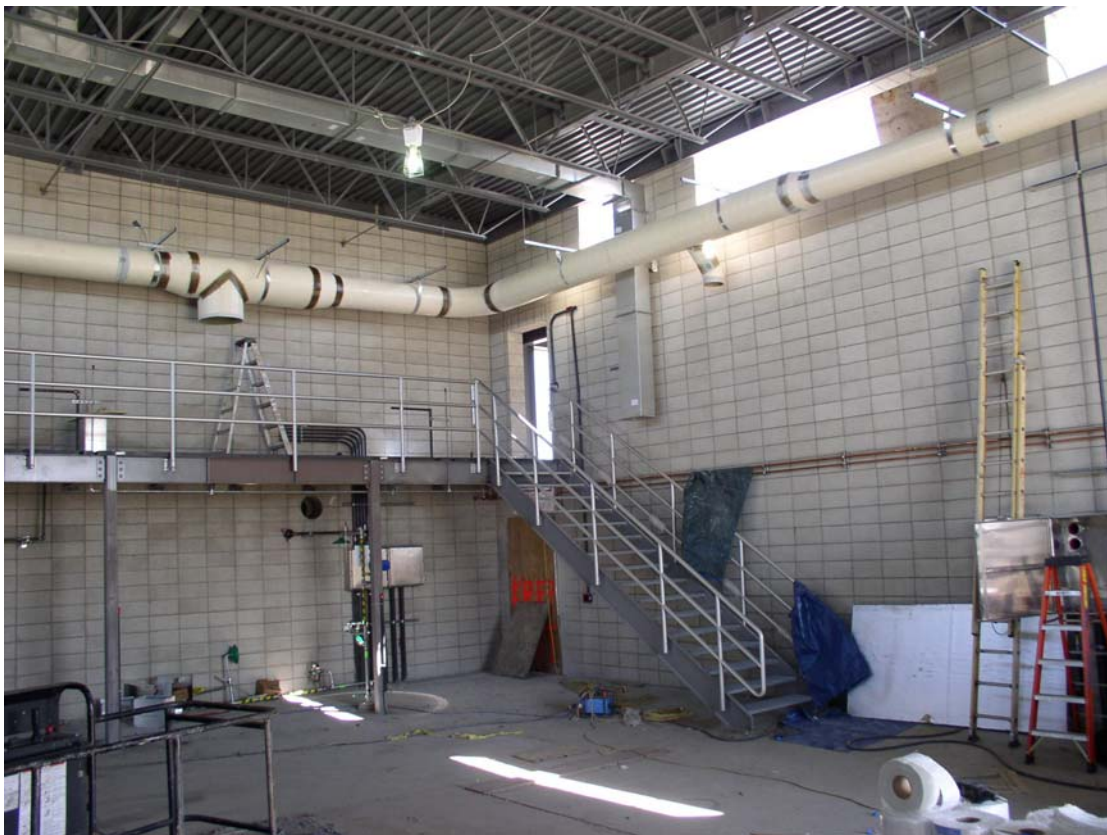
Figure 14: Mills chlorine containment facility
