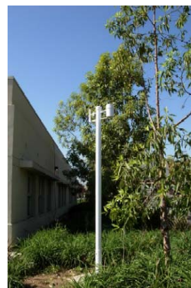
Smart Irrigation System (Sponsored by Pasadena)
