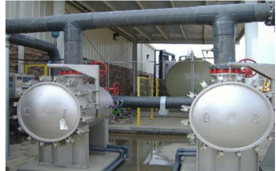
South Coast Water District, Capistrano Beach Desalter (Sponsored by MWDOC)
