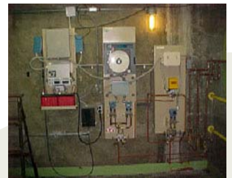
Water flow meter tied into AMR system
