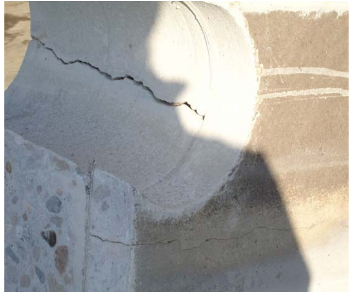
A cracked pipe at the third location.
