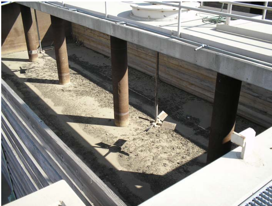
Figure 5: Modules Nos. 1&2 mixing equipment to be rehabilitated
