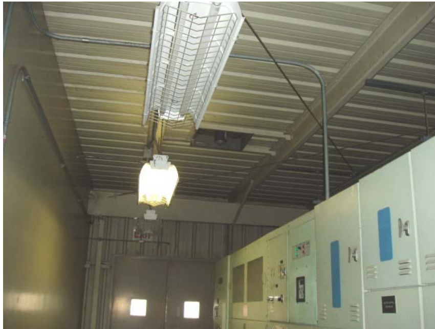
Figure 7: Interior of electrical building
