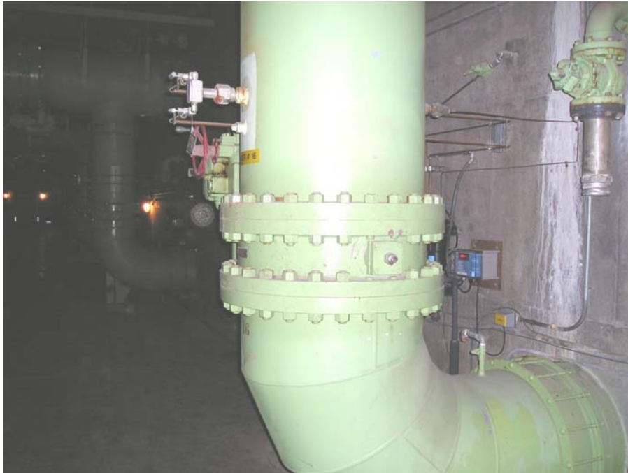
Figure 6: One of the Module No. 1 filter valves to be replaced
