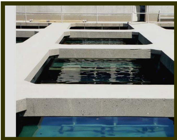
Weymouth Water Treatment Plant Replace Surface Wash Headers in Filter Building No. 1
