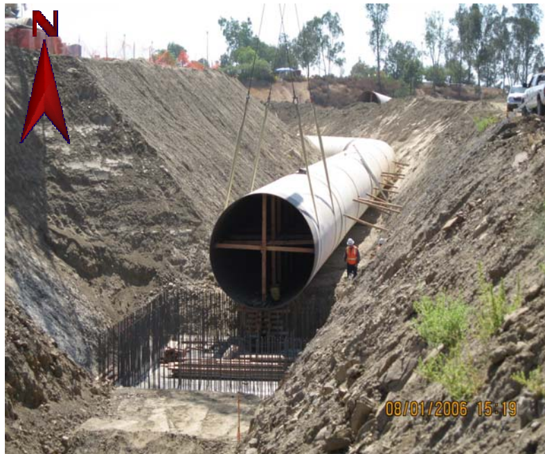
Figure 7: Skinner plant – Connection between Plant No.1 inlet pipe and contactor outlet channel
