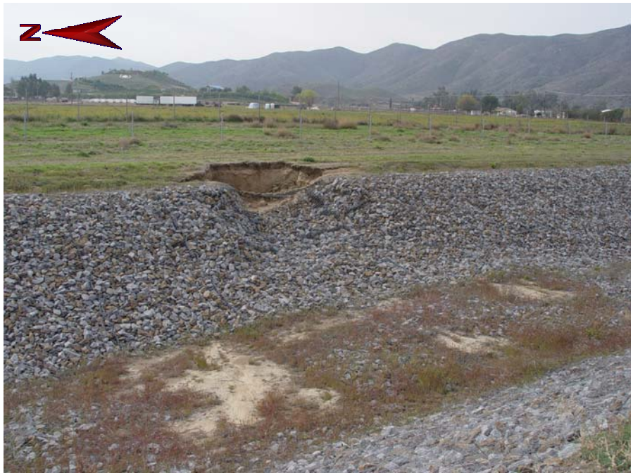
Figure 5: Storm run-off damage at St. Johns Canyon Channel
