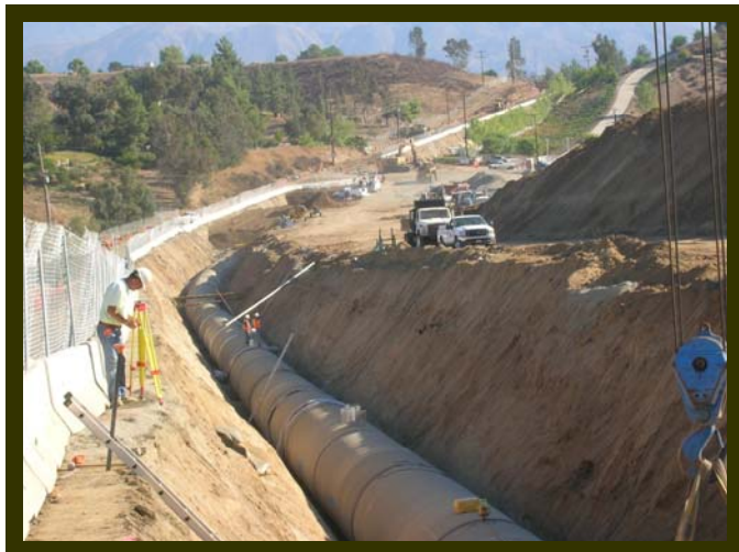
San Diego Pipeline No. 6
