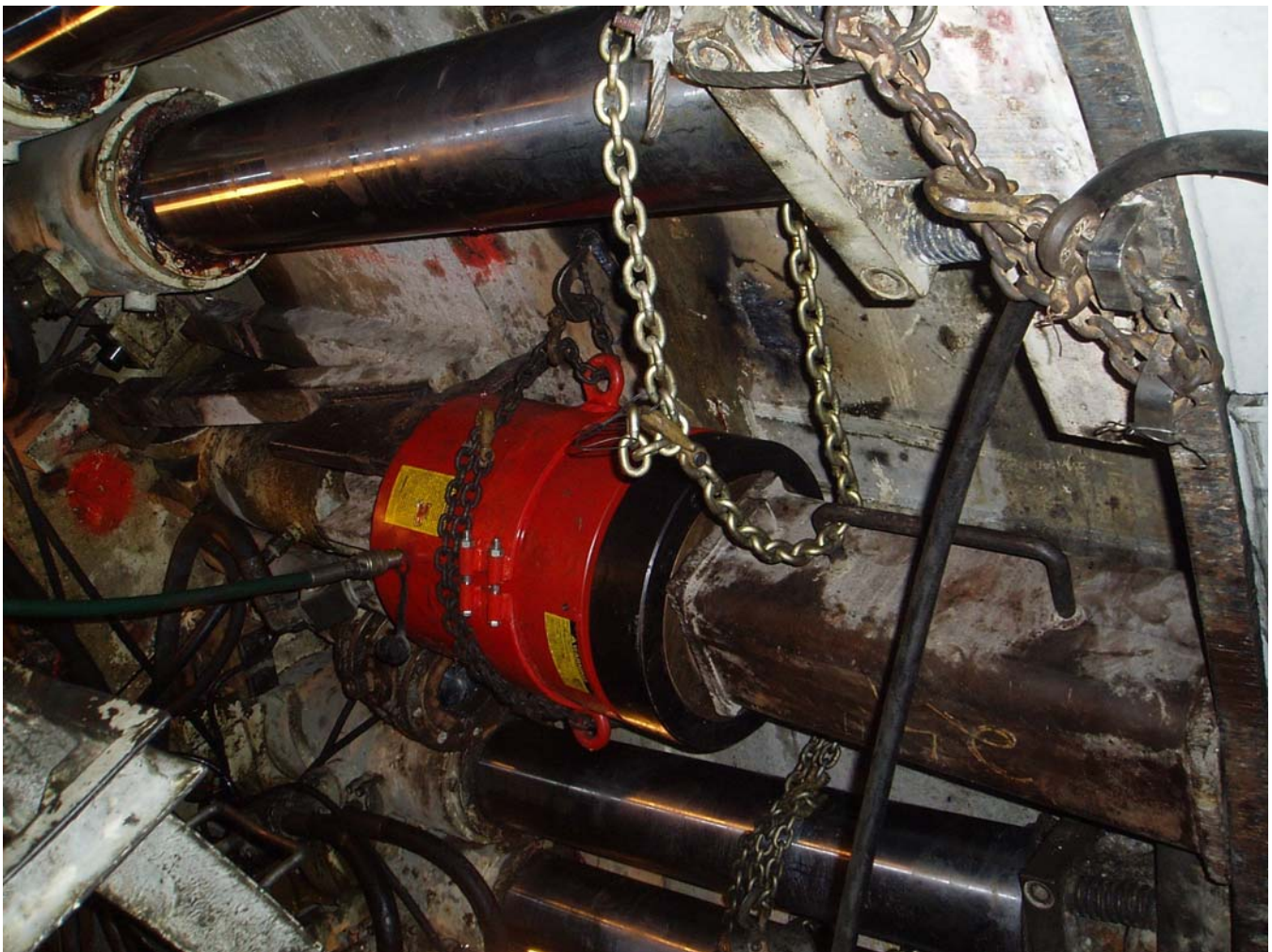
Figure 3: Using auxiliary jacks (560 ton each) to release the TBM shield from stuck position
