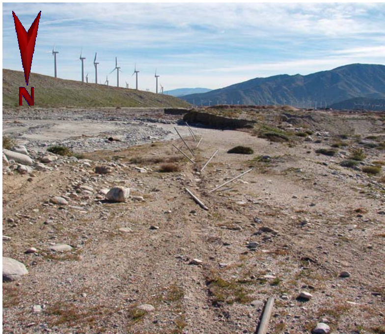
Figure 7: Damaged MWD fencing and protective berm along the Whitewater River, looking north
