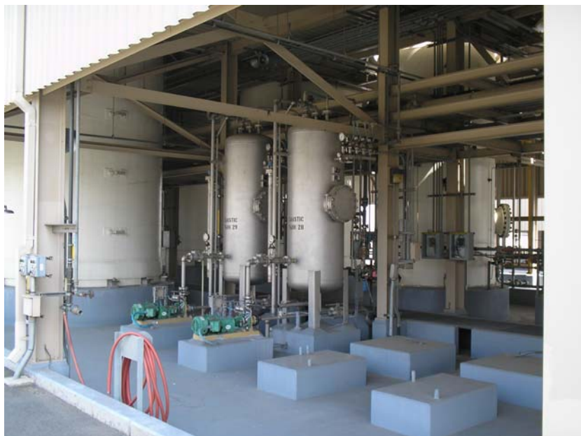
Figure 4: Mills Caustic Tank Farm
