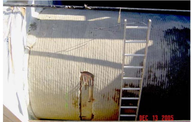
Santa Ana Valley Pipeline with exposed broken wires. If not repaired this condition could have resulted in a catastrophic failure of the pipeline. (Photo courtesy of DWR.)
