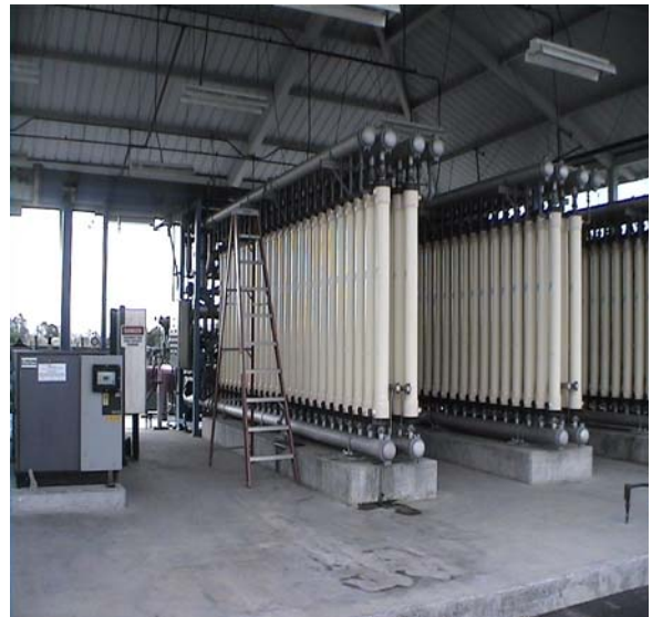
Alamitos Barrier Reclaimed Water Project (Micro-Filtration Station) (sponsored by Central Basin MWD)
