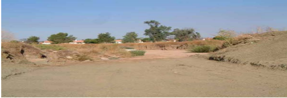
Figure 1: Salt Creek Channel 2005/2006 Rain Season Erosion
