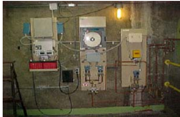
Water flow meter tied into AMR system
