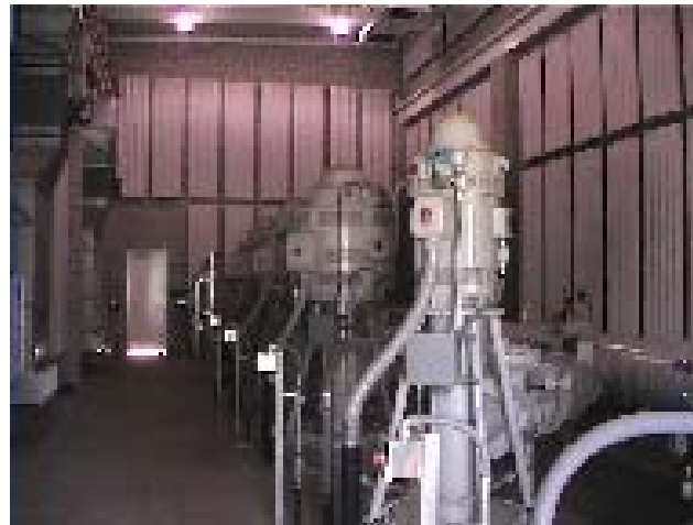
Escondido's Hale Avenue Resource Recovery Facility
